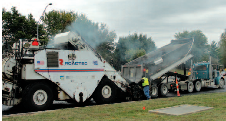
Mur-Len Road received a mill and overlay improvement as part of the City of Olathe’s 2011 Street Preservation Program. Olathe completed 45 lane miles of this maintenance during 2011. The projected mill and overlay maintenance needed in 2012 is 80 lane miles, based on the total number of lane miles in the network.
